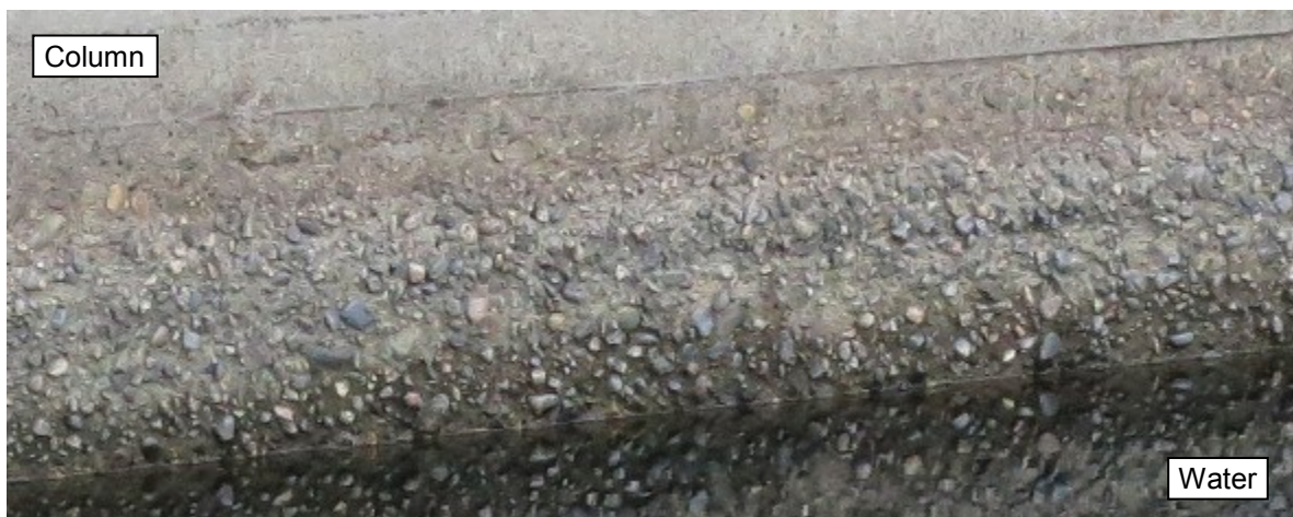
Figure 1: Coarse aggregate exposed at the waterline on the upstream face of a concrete dam. The water level was about 0.3 m lower than normal when the picture was taken.
